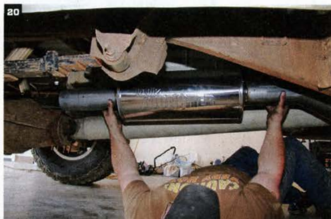
After the downpipe is installed, Bruner is able to install the rest of the stainless steel, 4-inch-diameter exhaust system. Using the supplied clamps and hangers, everything lined up perfectly under the truck.
