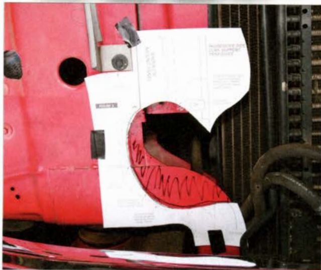
Next, Bill used the supplied templates provided by Banks to make exact markings where the intercooler pipes would fit into the core support.
