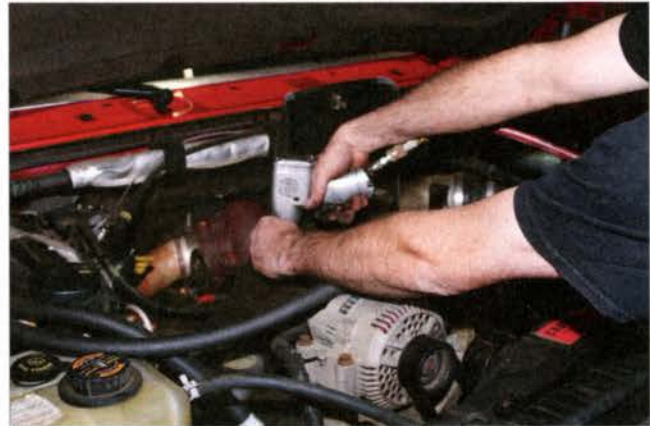
We had to remove the stock fuel filter cover (door) to allow room for the pipes.
