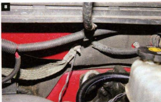
The SpeedBrake ground is connected to the ground stud on the firewall near the brake master cylinder, where it will join a factory ground strap.
